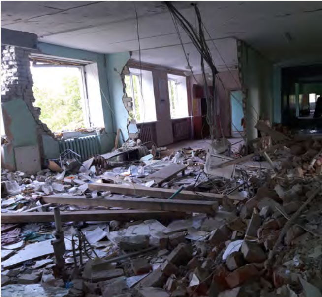
Top: Damage to the exterior of the Trostianets City Hospital. Photo captured by the Ukrainian Healthcare Center in August 2022.
