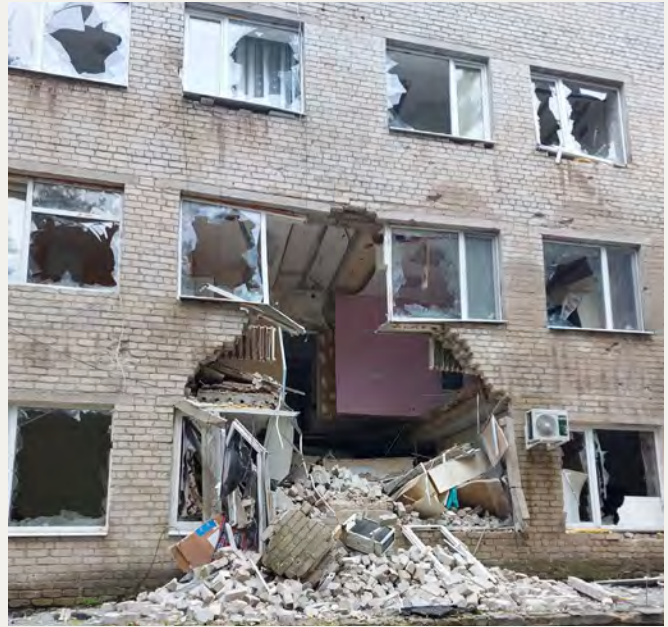
Severe destruction of one of the buildings of the Balakliia Clinical Multiprofile Intensive Care Hospital, which was allegedly hit by a tank. Photo captured by the hospital's medical personnel in September 2022.
