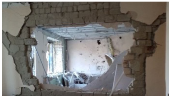
Trostianets City Hospital was struck five times in March 2022. Photo captured by the Ukrainian Healthcare Center during a site visit on August 11, 2022.
