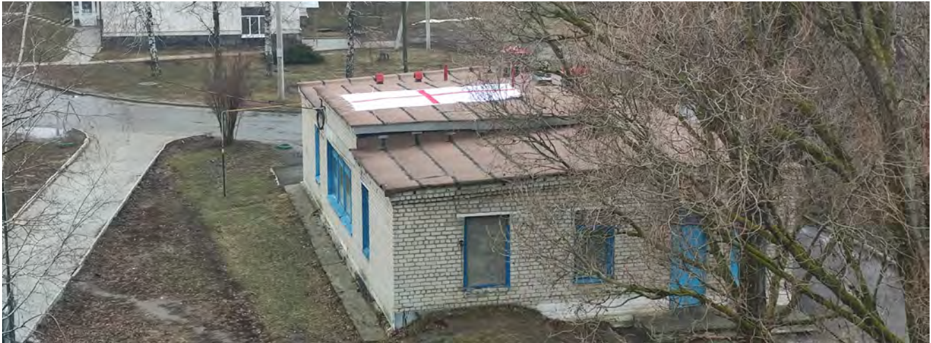
A technical building at the Iziium Central City Hospital, which was damaged in at least three attacks in March 2022, showing the red cross placed on its roof to indicate its status as a medical facility. Photo captured by hospital director Dr. Bohdan Berezhnyi in Feb/Mar 2022.
