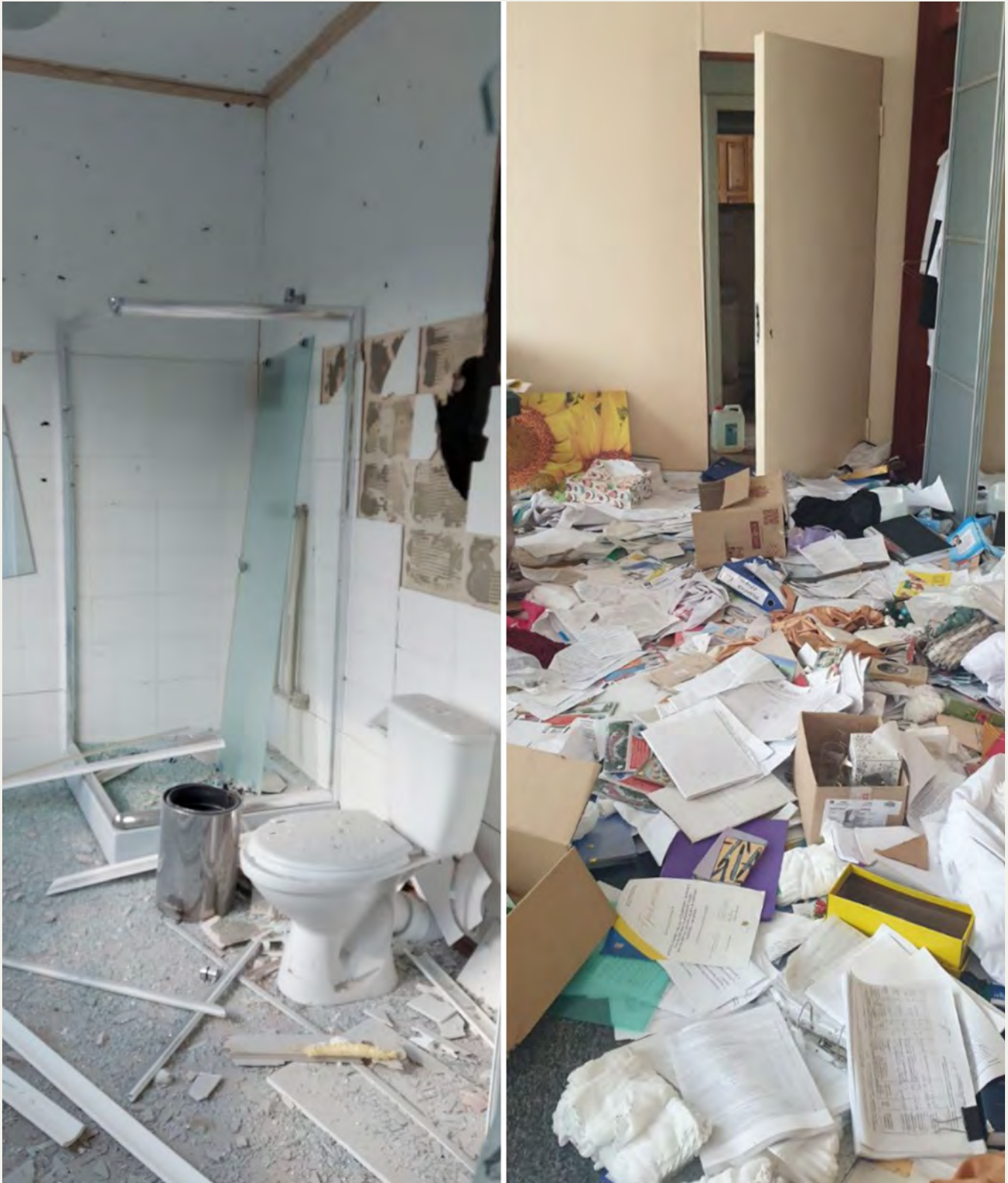
Above: Vandalized premises of the the Balakliia Clinical Multiprofile Intensive Care Hospital. Photos captured by the hospital's medical personnel in September 2022.
